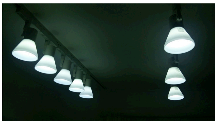
FIGURE 4. Ceiling light fixture arrangement.
